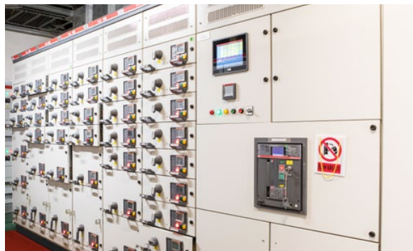
MNS Digital Low Voltage Switchgear in ABB Xiamen Hub
