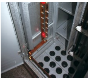
Ground protection bar and neutral bar
