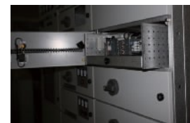
Moveable switchgear cabinet
